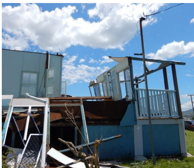
Tropical Cyclone Marcia caused significant damage to property in Yeppoon, Queensland due to its severe winds.
