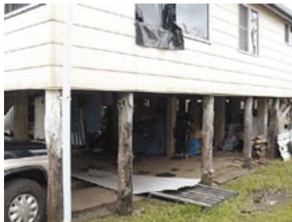
Wind impacts were ‘patchy’. This 90 year old house in Mourilyan survived with a couple of damaged windows. Photo: Douglas Goudie
