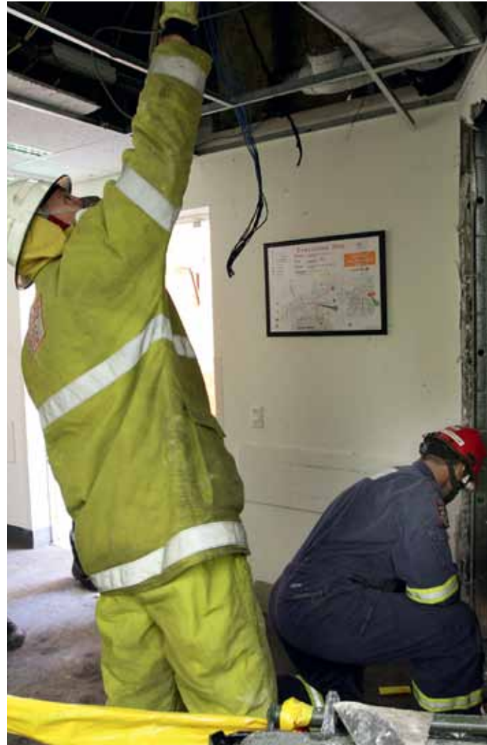
Firefighters assess damage inside Armadale-Kelmscott Memorial Hospital. Photo courtesy Community Newspaper Group .
