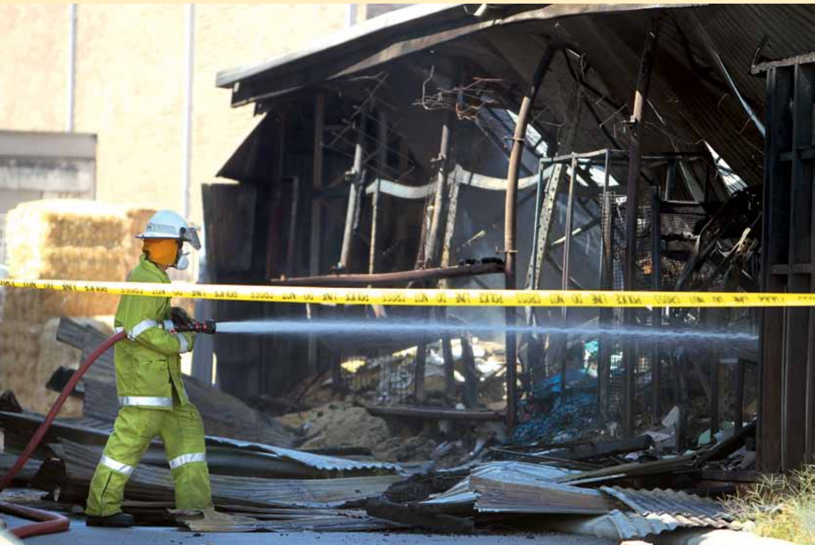
The collapsed roof and large amount of product at the store made access to the seat of the fire difficult for crews. Photo courtesy of The West Australian .
