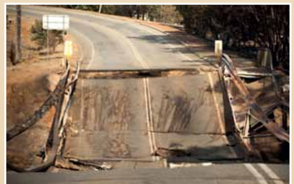
The 76 year old Buckingham Bridge collapsed in the bushfire.
