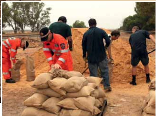
SES volunteers and inmates from Greenough Regional Prison fill sandbags at Walkaway. Photo courtesy Geraldton Guardian .
