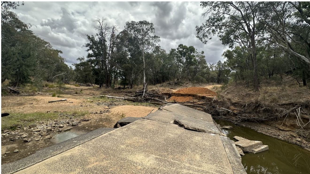
Figure 2: Road damaged by flooding in the Warrumbungle local government area.
