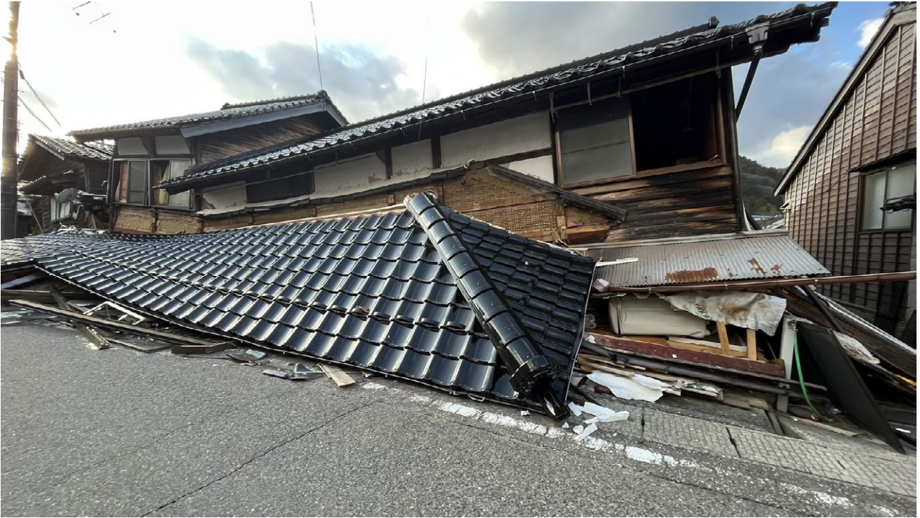
In 2024, the earthquake on the Noto Peninsula caused extensive damage and collapsed buildings.
