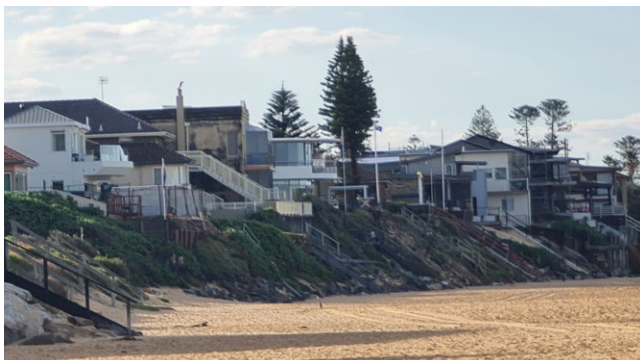
Legacy development on the eroded beachfront of Wamberal, New South Wales.
