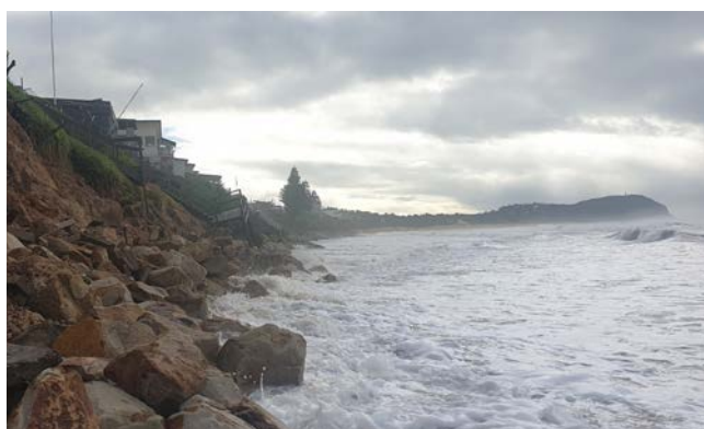
Storm surge exposed rocks and damaged infrastructure at Wamberal Beach, New South Wales, July 2020.
